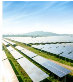
Array Power Station
