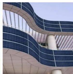
BIPV Building Integration
