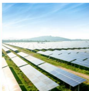
Array Power Station
